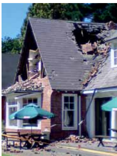
2011 Earthquake damage on Clubhouse
